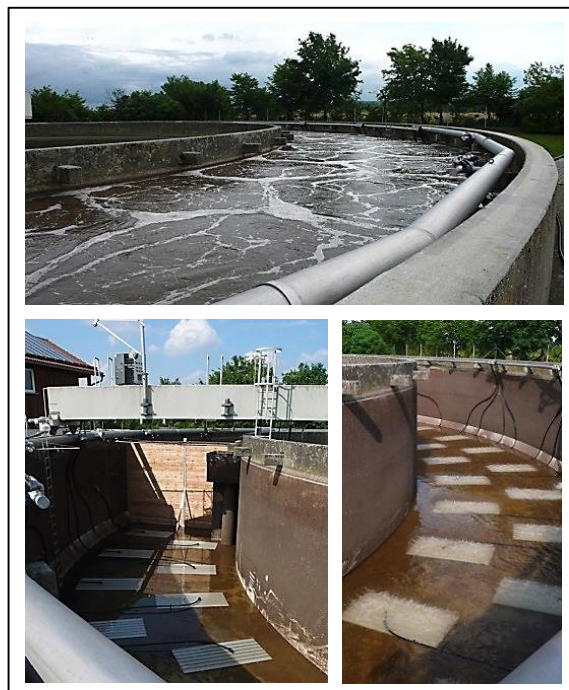
Figure 1: Activated sludge tank of WWTP Adelsdorf during and after installation of the MESSNER Aeration Panels.
